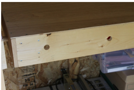
Photo 2- Note the one inch holes drilled every 12 inches.
